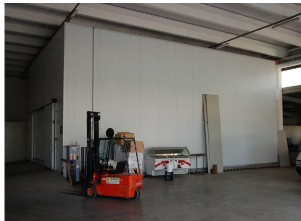
Fig. 4 Freezer cell installed and in use
