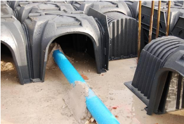
Fig. 1 Detail of plumbing under Modulo
